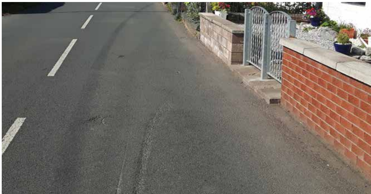
Gouges in the road surface on Glencaple Road from tractor and trailer which came round the bridge corner too fast. Also note the new walls (to replace originals destroyed at the time)
